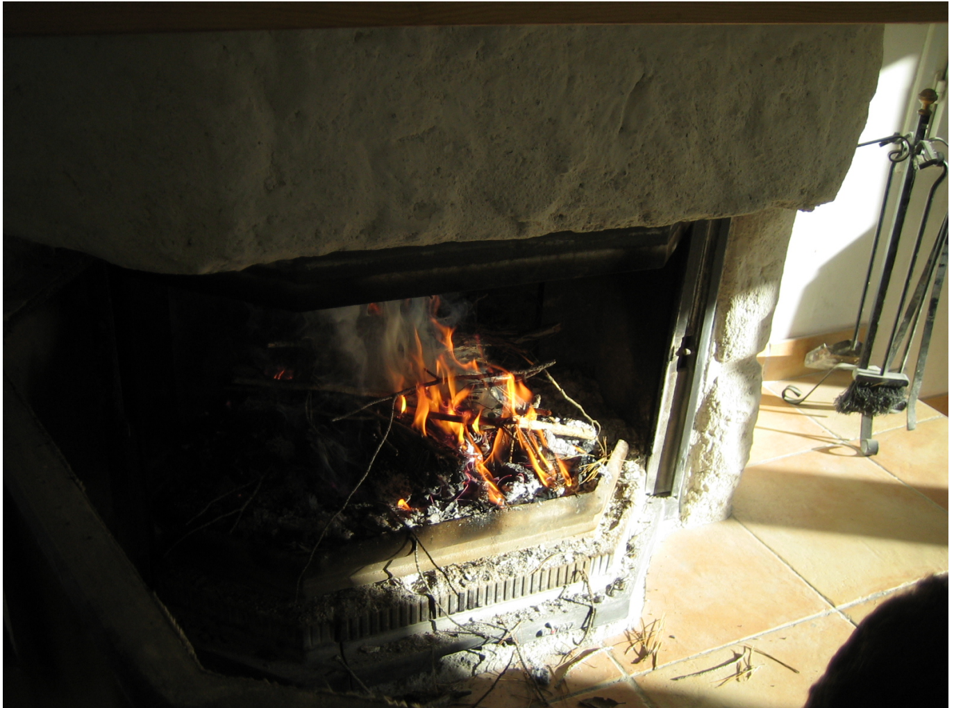
The oldest decentralised heating technology.
